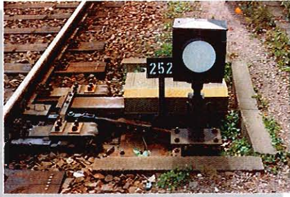
Prototypical built up roadbed area at the location for the switch linkage
